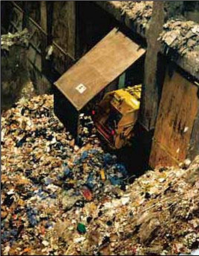
Måbjergværket has two boilers for the incineration of waste, and the combustion capacity is 10 tons of waste an hour.
