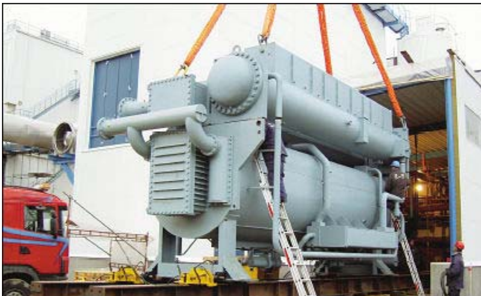
Lifting the absorption heat pump, with the help of which it will be possible to extract extra energy for the district heating network.
