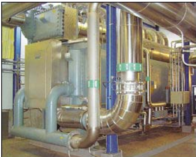
The absorption heat pump in place. The installation has surpassed the expectations of Karlstads Energi.
