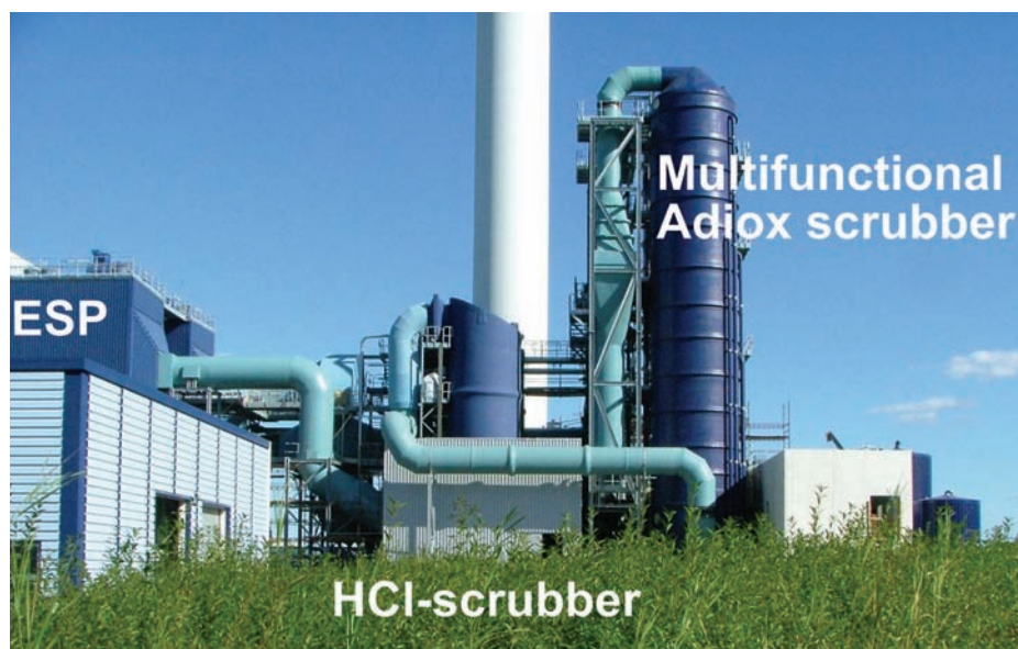
Figure 2: Adiox has been in operation as a primary dioxin removal system at Måbjergværket (Denmark) since the fall of 2004. All measurements are far below the 0.1 ng TEQ/Nm 3 .
