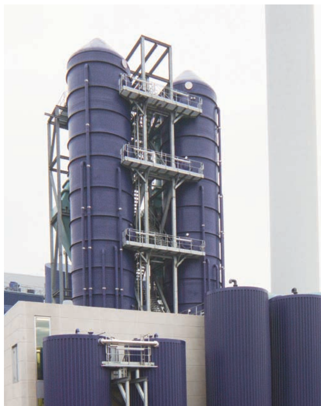
Multi-functional scrubber at Måbjærgværket in Denmark as a primary dioxin removal system with dioxin removal rates in excess of 99%.
