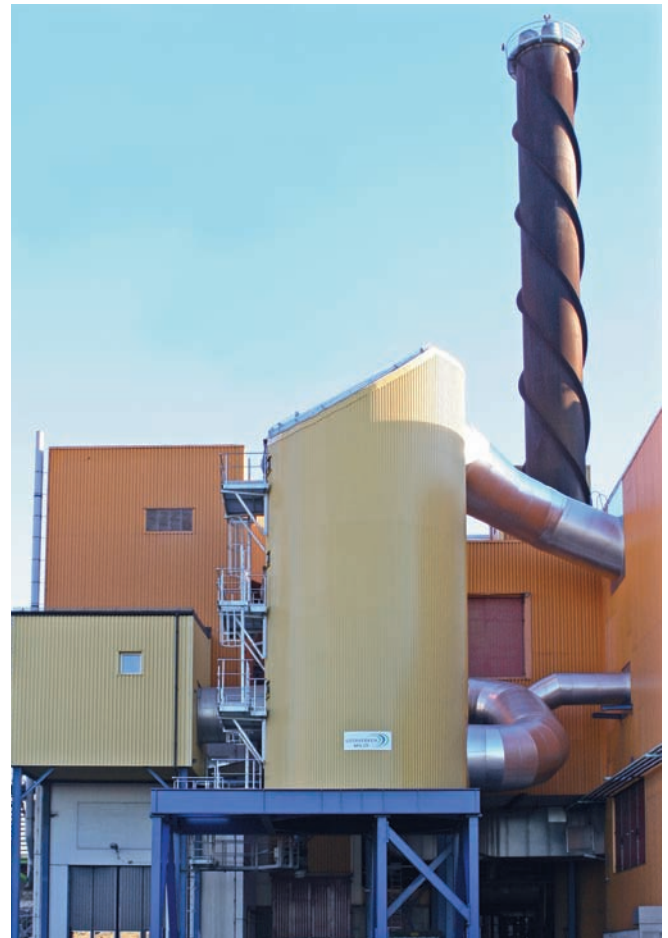
Dry ADIOX® absorber installed after fabric filters at a waste incineration plant at Gärsåderverket in Linköping, Sweden.
