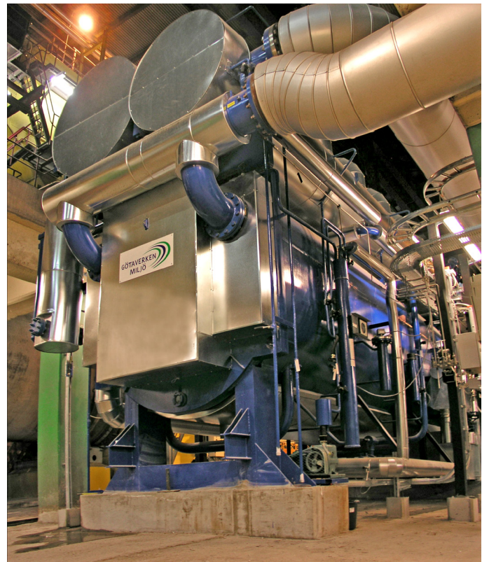
Absorption heat pump at Vestforbrænding, Denmark.
