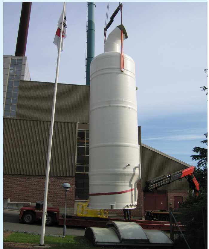
The wet scrubber condenser at Aars Varmeværk when lifted into the building in June 2011.
