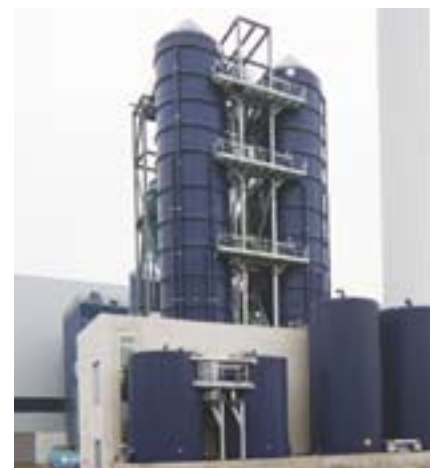
The two multistage scrubbers at Måbjergværket in Holstebro, Denmark.
