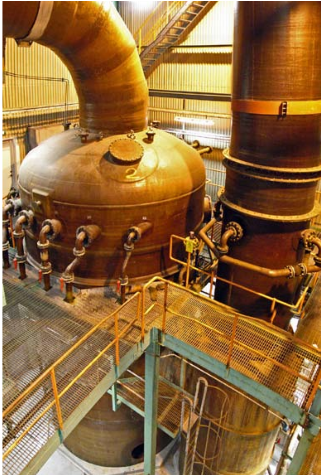
Scrubber and quench at line 3, Renova. These are to be replaced in 2008.
