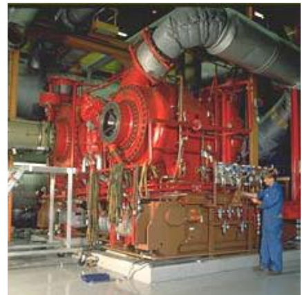
Compressor heat pumps at Rya, Gothenburg.
