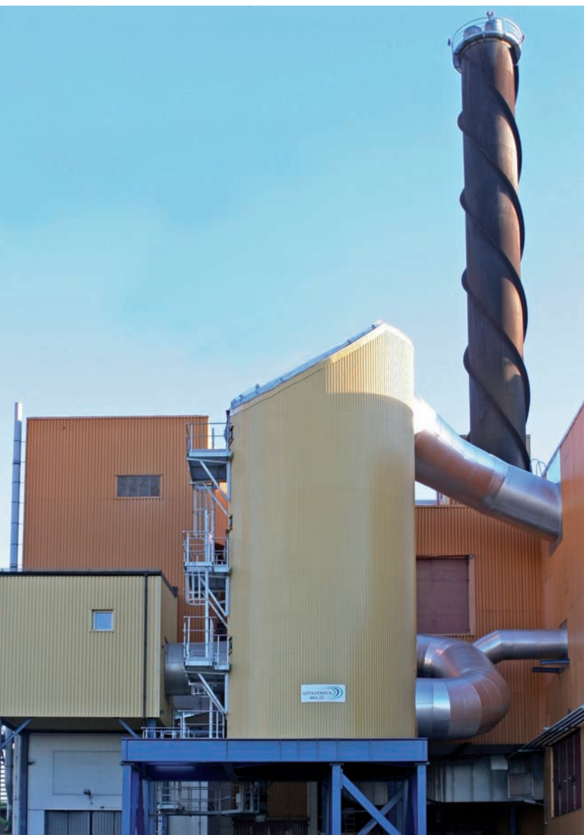
The dry ADIOX® absorber at Gärsstadverket.
